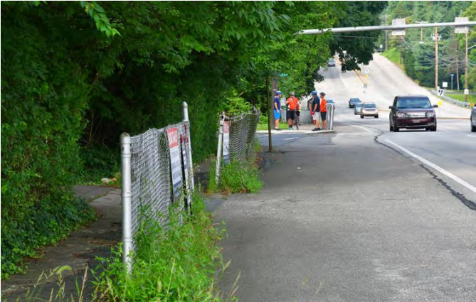
Figure 17 – Deficient sidewalk and fencing, Cumberland Boulevard northbound looking south towards 24 th Street
