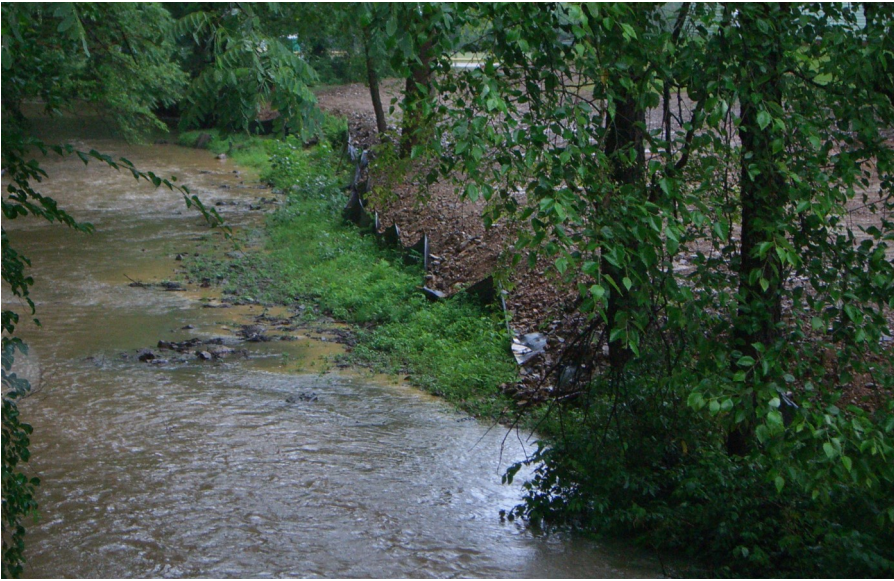
Unattended to Erosion Prevention Measures, June, 2006
