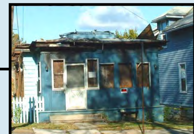
Poor: Structures with interiors that have significant exposure to the outdoor elements. Missing windows and dilapidated rooftops are some of the more common examples. These structures are typically vacant and in some cases have evidence of fire damage.
