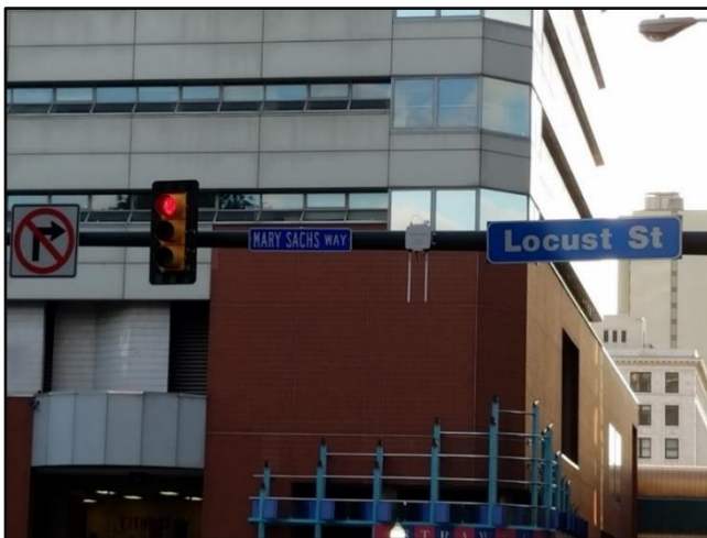
DSRC radio installed on traffic signal mast arm
