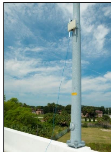
Highway pole mounted DSRC
