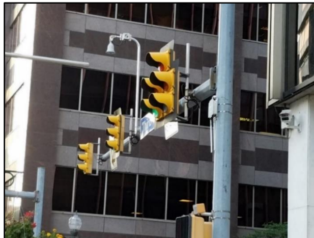
Intersection signal pole mounted (not enough room on the signal mast arm)
