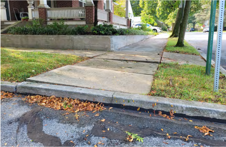
A Hummelstown sidewalk with no curb ramp
