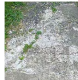
Major Spalling/ Scaling
