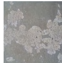
Moderate Spalling/ Scaling
