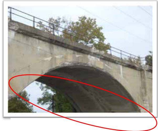
Figure 10: Spalled Concrete Visible on CAT Bridge
