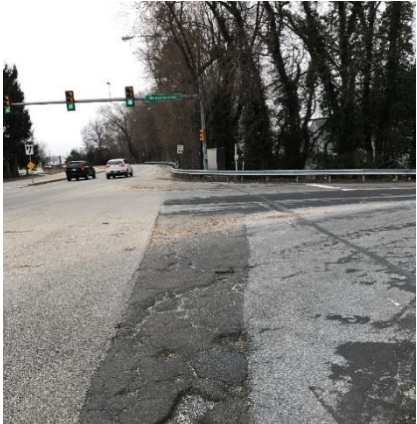
Figure 12 – Existing poor crosswalk conditions, Brentwater Road at Cumberland Boulevard
