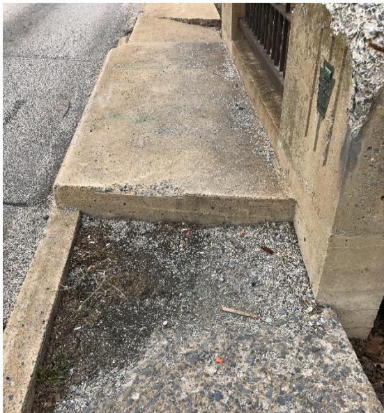
Figure 3 – Damaged sidewalk at culvert, 32 nd Street northbound, south of Chestnut Street, looking north
